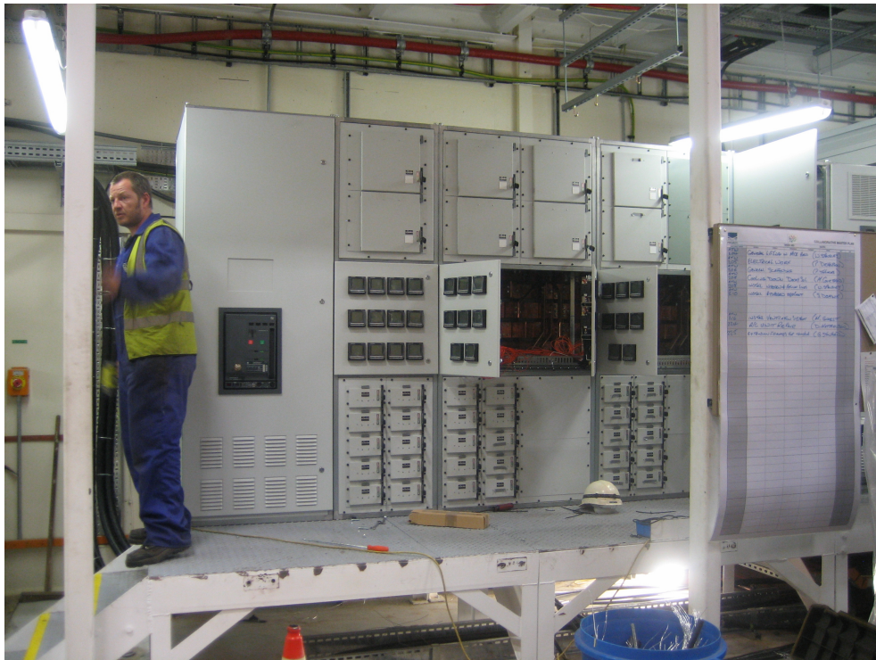
Figure 42: This photograph of part of the substation in the MICE hall clearly shows that a significant amount of electronics has been mounted in the front panels.
