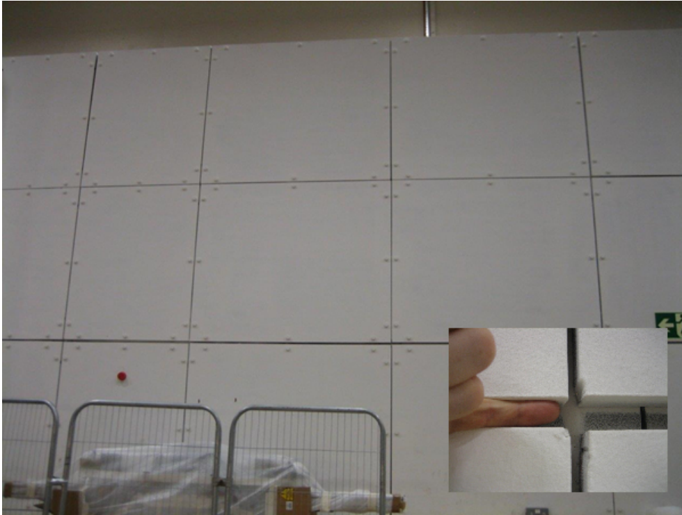
Figure 36: Photograph of the north shield wall. The gaps between the plates can be clearly observed.
